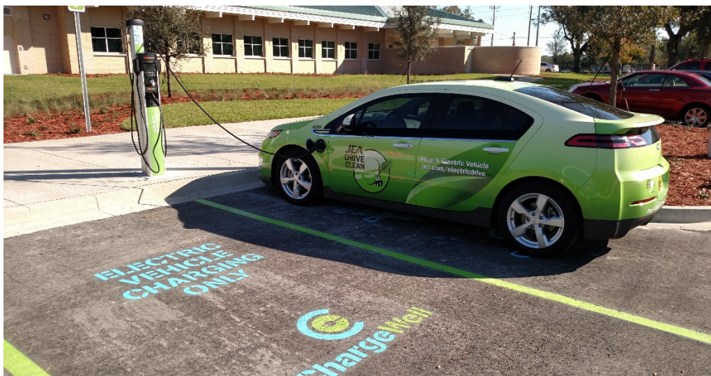
FIGURE 3: CHARGEWELL EV CHARGING STATION AT THE NORTH FLORIDA TPO'S OFFICES IN JACKSONVILLE
