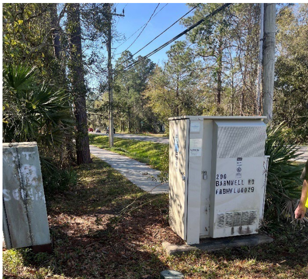
End of Existing Sidewalk in the Vicinity of Barnwell Circle. Photo Source: Project Team.
